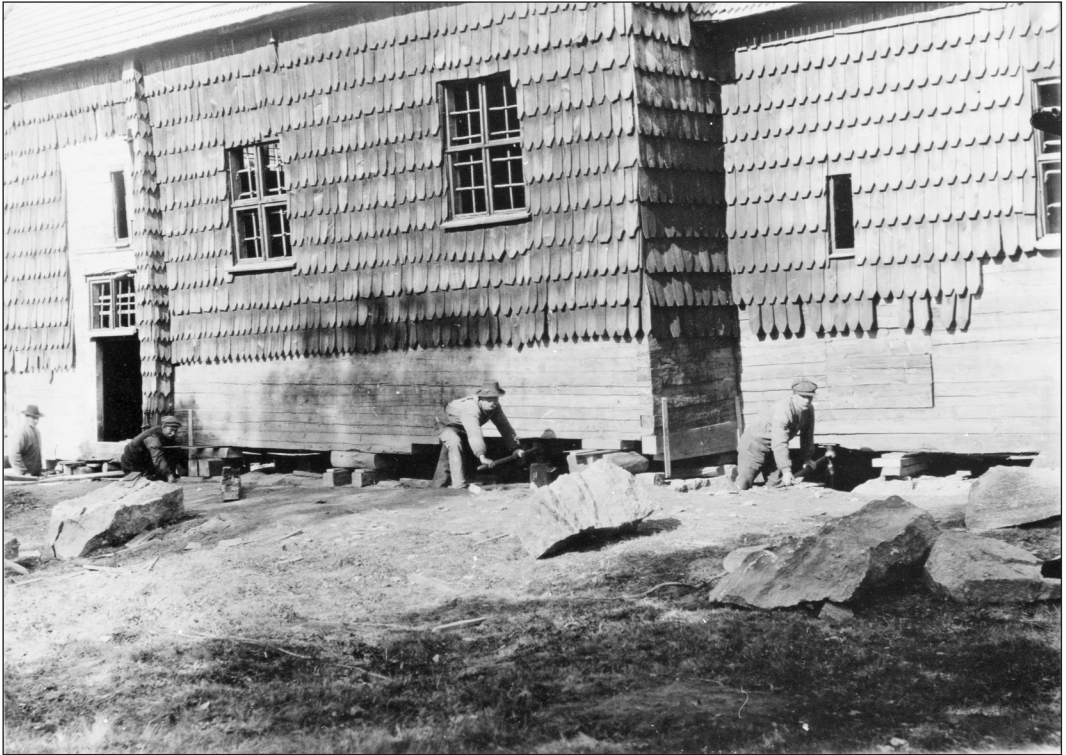
Figure 2: The church of Södra Råda was restored at several times around the turn of the century 1900. Here, the original southern entrance has been uncovered and the craftsmen are lifting the timber structure to replace the sill. (Photographer and year unknown. Source: Swedish National Heritage Board. Photo id. 3180-020. Public Domain)
